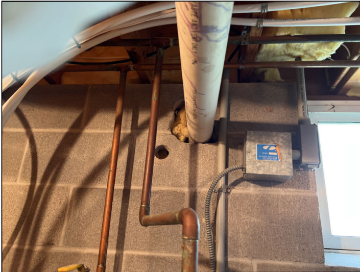
Gaps noted around water heater vent pipe on the inside and outside of foundation. Recommend sealing
