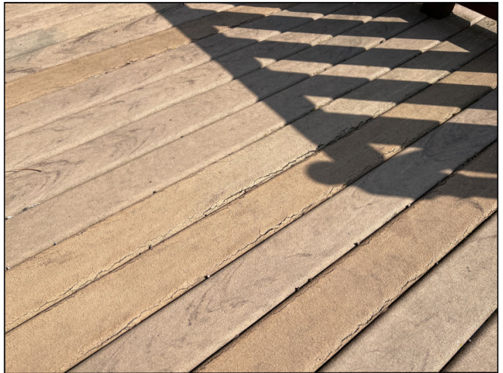
Cracking/warping composite decking. Recommend replacing decking
