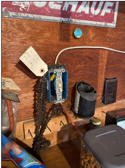
Missing cover plates observed, suggest installing for safety.
