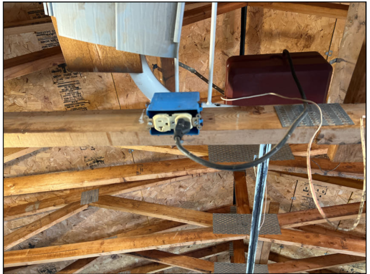
Missing cover plates observed, suggest installing for safety.
