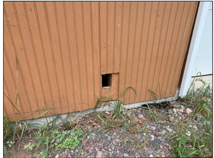
Hole in siding at back of garage. Recommend repair
