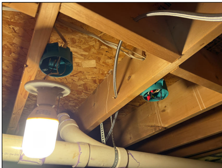
Open junction boxes/unattached fixtures were observed in basement utility room which is a safety concern. Recommend installing proper covers and/or fixtures as needed, for safety.
