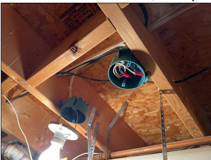
Open junction boxes/unattached fixtures were observed in basement utility room which is a safety concern. Recommend installing proper covers and/or fixtures as needed, for safety.
