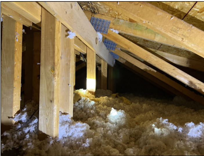
Appeared functional with no deficiencies noted at the time of the inspection.
