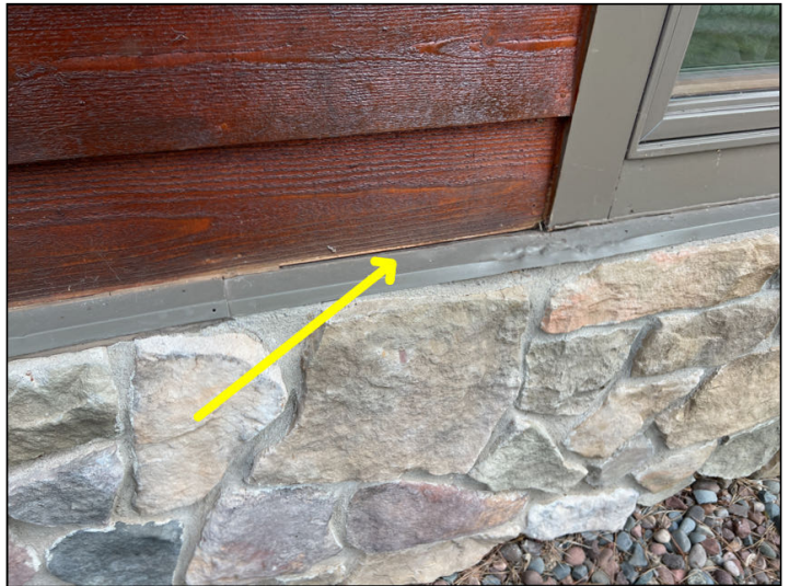
Caulk/seal gap at siding/stone transition flashing to right of front door
