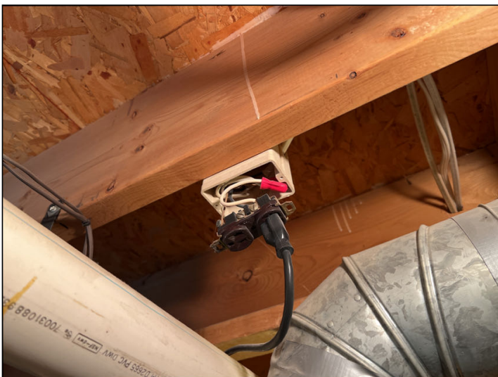
Open junction boxes/unattached fixtures were observed in basement utility room which is a safety concern. Recommend installing proper covers and/or fixtures as needed, for safety.
