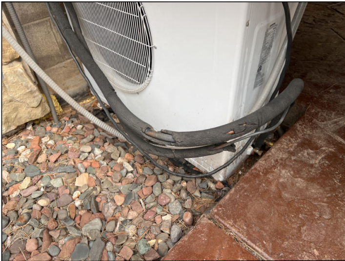
The insulation is missing or damaged at exterior refrigerant line. Recommend replacing insulation for efficiency
