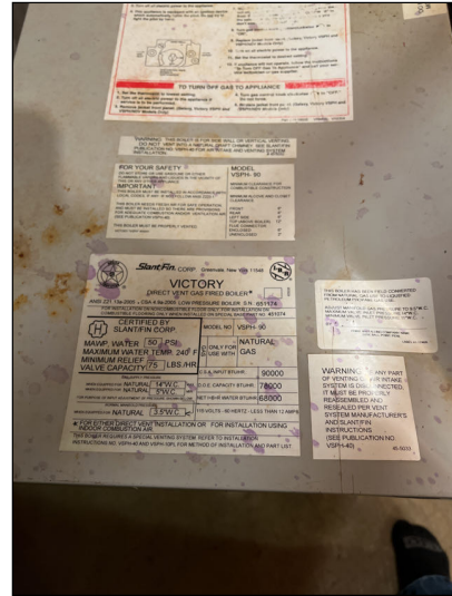
Furnace/Boiler date of manufacture: Estimated post 2005
