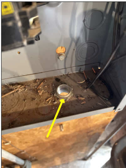
Knockouts need snap-in caps inside panel box. Should be installed to keep mice out of panel box and to avoid potential electrocution hazard.
