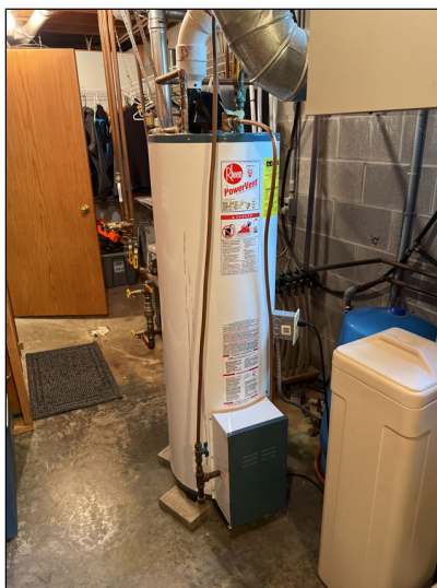
Appears functional with no deficiencies noted at the time of the inspection.
