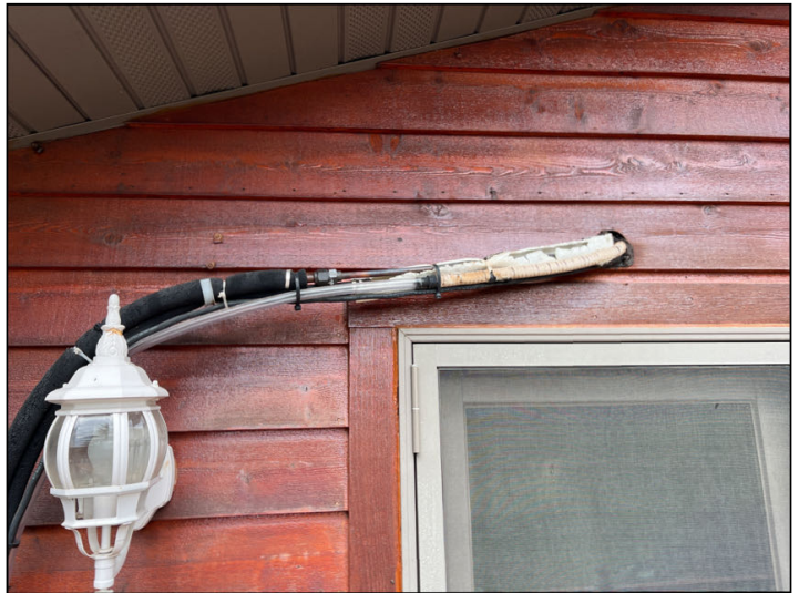
The insulation is missing or damaged at exterior refrigerant line. Recommend replacing insulation for efficiency
