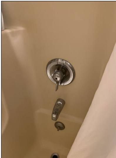
Hot/cold reversed plumbing observed on main floor shower valve
