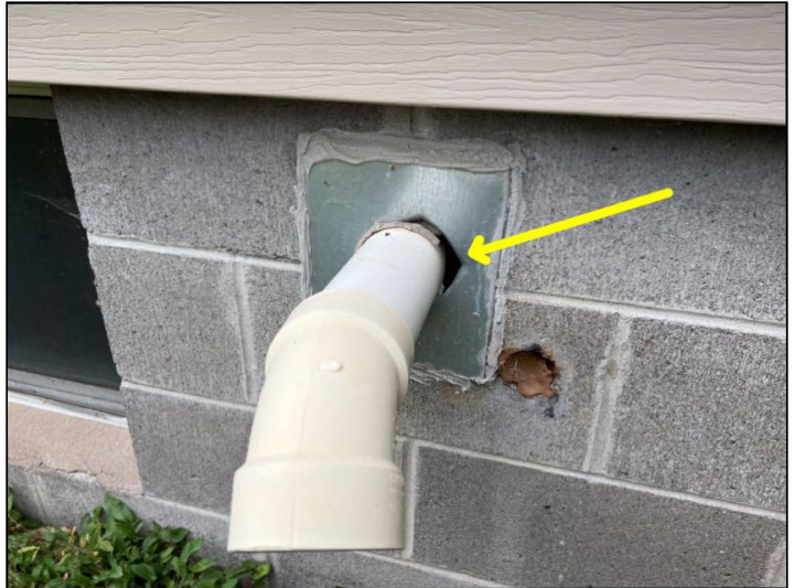
Gaps noted around water heater vent pipe on the inside and outside of foundation. Recommend sealing
