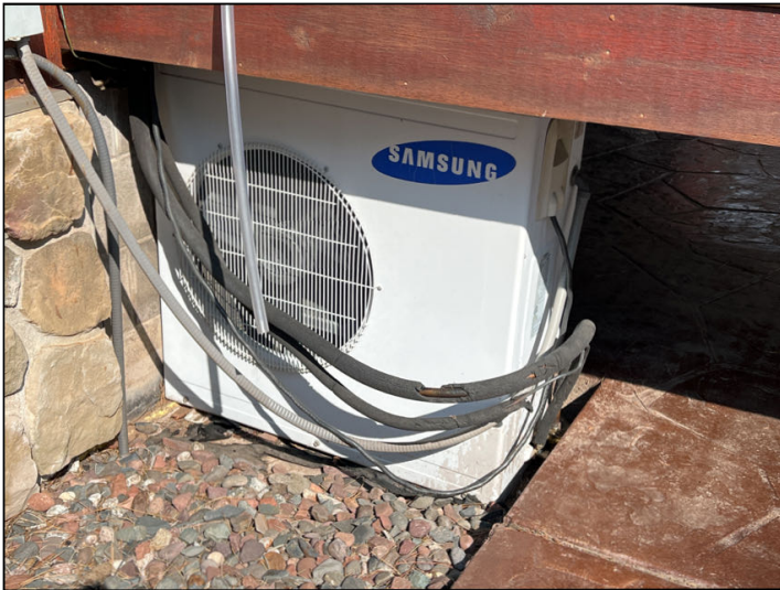
Appeared functional with no deficiencies noted at the time of inspection.
