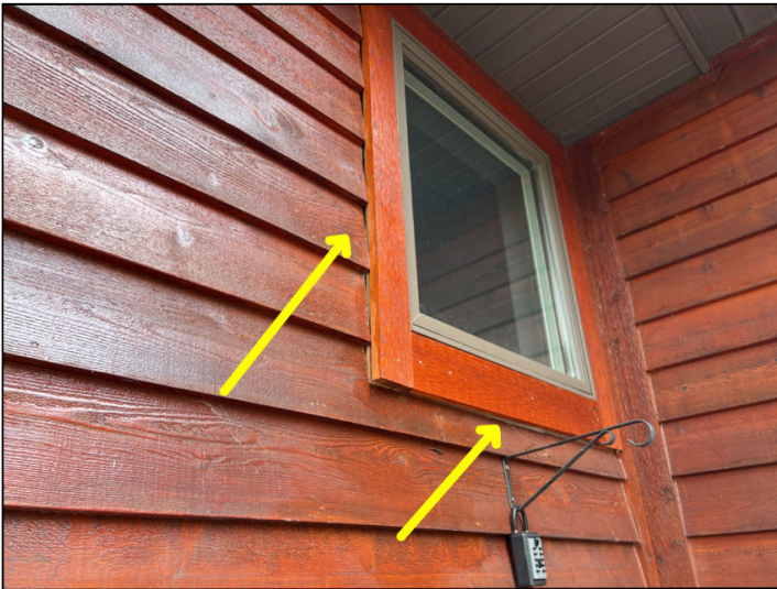
Caulk and seal all gaps, cracks and openings. Window at left of front door needs caulking
