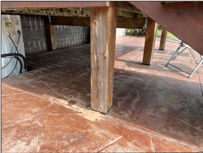
No permanent deck footings noted. Floating decks are susceptible to heaving.
