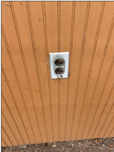
Weatherproof cover missing on outlet on front of garage. Install for safety
