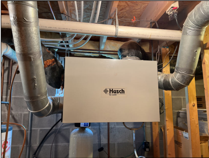
The air exchanger appears to be functional.
