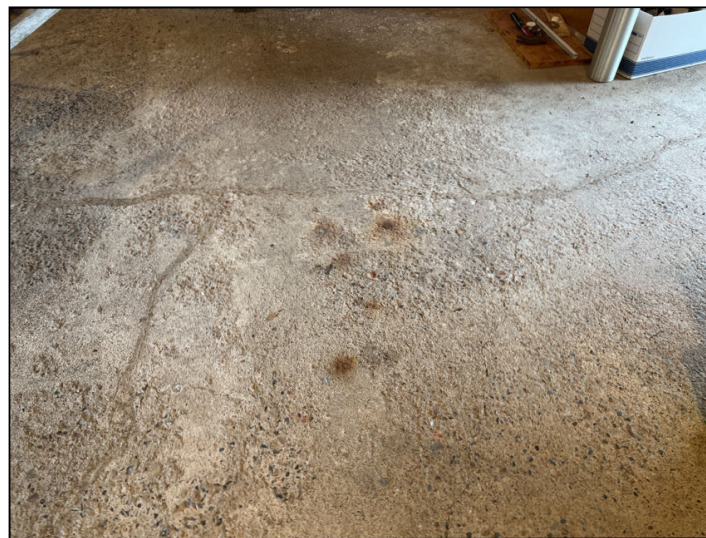
Common cracks noted. Minor spalling noted.
