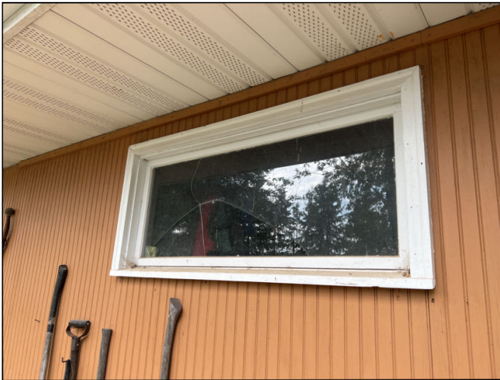
Cracked/broken glass-left side window on garage
