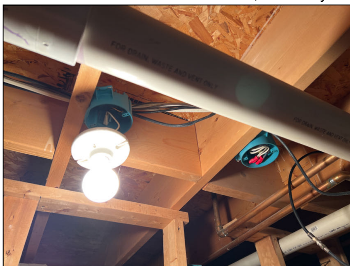
Open junction boxes/unattached fixtures were observed in basement utility room which is a safety concern. Recommend installing proper covers and/or fixtures as needed, for safety.
