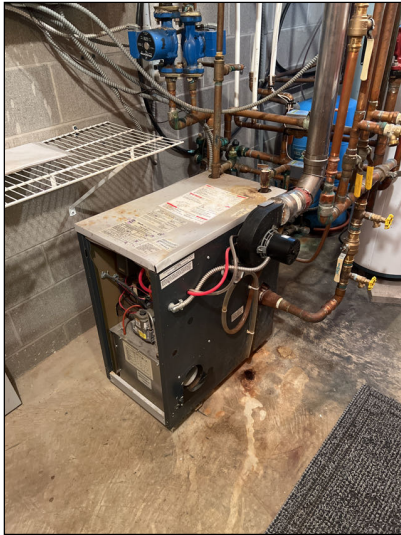
Appears functional with no deficiencies noted at the time of the inspection.
